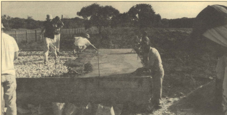
Pouring a 20 x 24 foot slab of concrete for the second house took seven hours.
